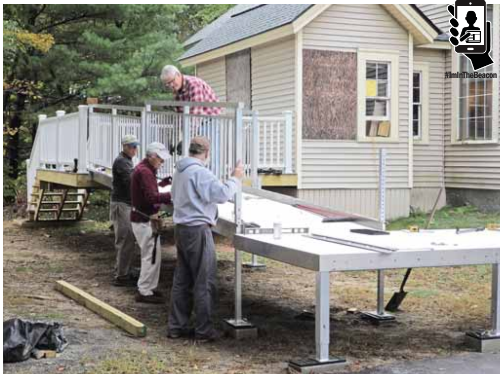
The project to build an access ramp to the Hub building, as part of the Capital Campaign, is underway. Shown at work are Hub volunteers Doug Phelps (on ramp) and Steve Darling, Harvey Pine, and Ken Wells. Photo: Larry Chase
