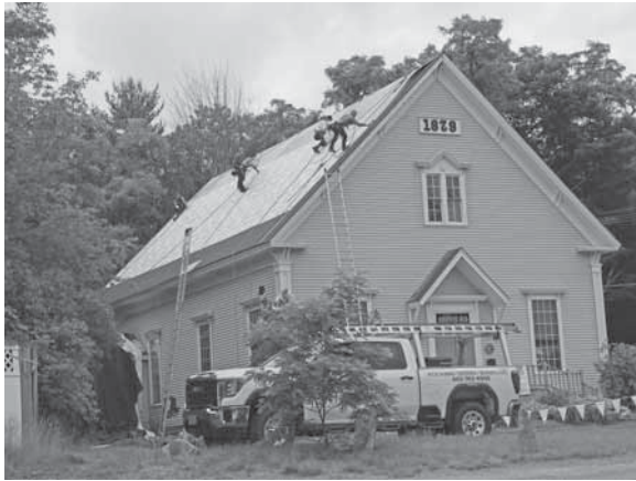
A major roof repair was completed earlier this summer as part of the Hub’s Capital Campaign projects. Photo: Larry Chase
