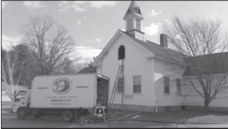
S hakes to Shingles continues work on the energy upgrades to the Andover Town Library. In November they filled in gaps and added R30 cellulose over the old section of the attic. Photo: Charlie Darling
