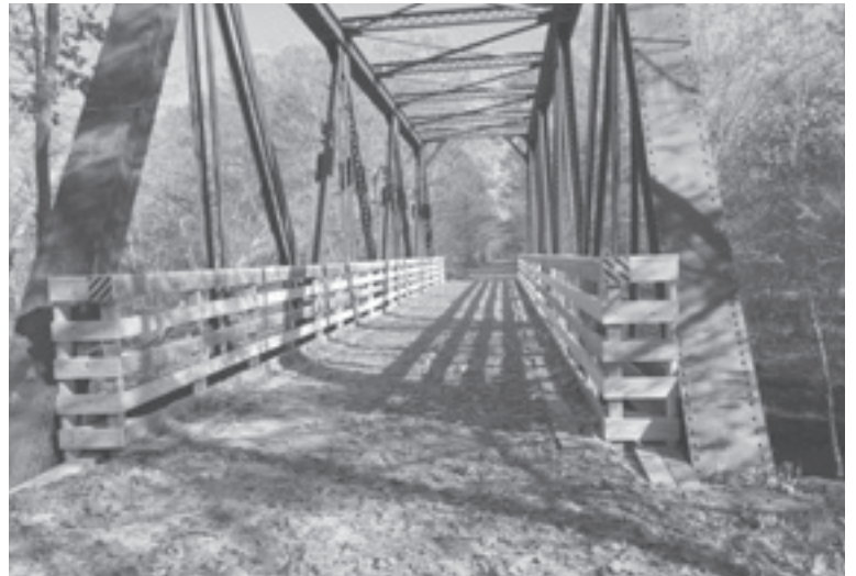
Rodney Judkins of Lakeview Construction in Franklin completed significant repairs on the truss bridge south of the Andover ball field. Some of the pressure treated rails were used elsewhere as temporary fixes and were reused here as planned. Notice that the bridge ends were boxed in by railings to cover the void that extended beyond.
