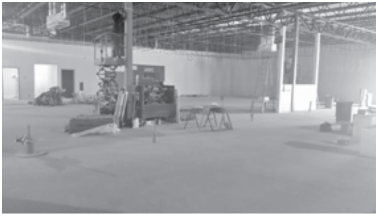
With the exterior nearly finished, work has turned to the interior of the new Belletetes retail store at Ten Penny Lane, across the street from the current retail location and attached to their Millwork Showcase. The big move should happen in early February, with a grand re-opening celebration to be planned for some time in the spring.
